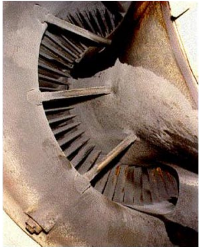
1. Don't let this happen at your plant. Severely fouled bellmouth and blading on a 35-MW engine operated in an industrial environment dramatically reduced GT performance
